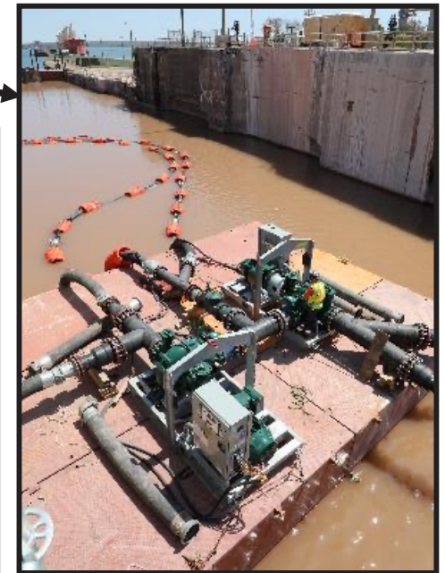
Hydraulic pump used to dewater construction site on barge in Davis Lock
