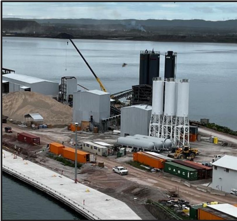
Expanded concrete batch plant
