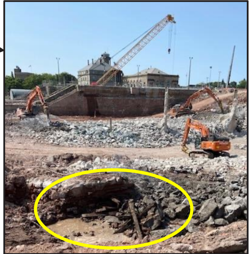
Exposure of century old Sabin Lock timber cribbing
